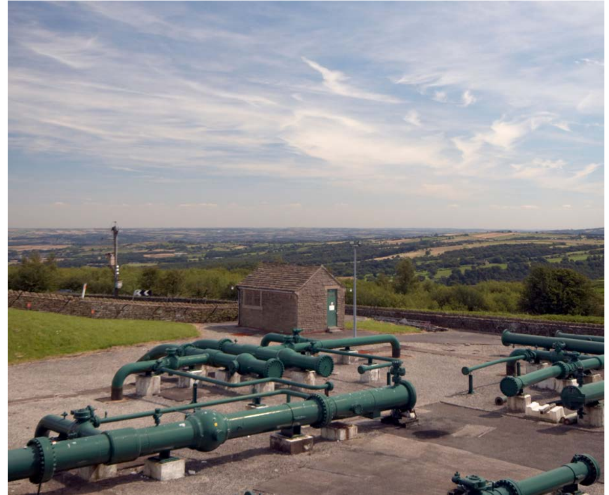
High pressure gas main compound, Derbyshire, UK
