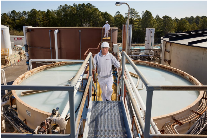
A wastewater treatment plant at SPI Pharma's manufacturing site in Lewes, Delaware, United States
