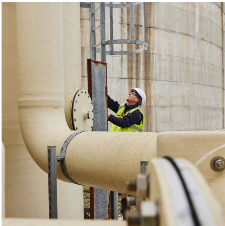
Anaerobic digestion plant at AB Mauri's site in Hull, UK
